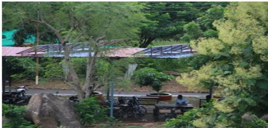
Installation of solar panels for the solar lighting system in GGITS , Parking area
