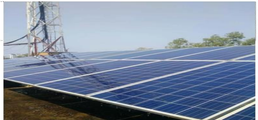
Real Time Data Acquisition System for 256 kW Grid Connected Solar Plant
